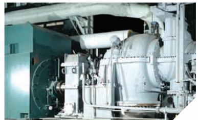
9 MW turbine generator set installed at a university in the midwestern United States.
